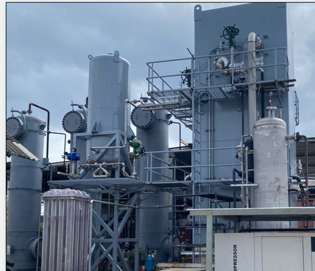
Saryozek Phase 1 LNG Liquification Facility
