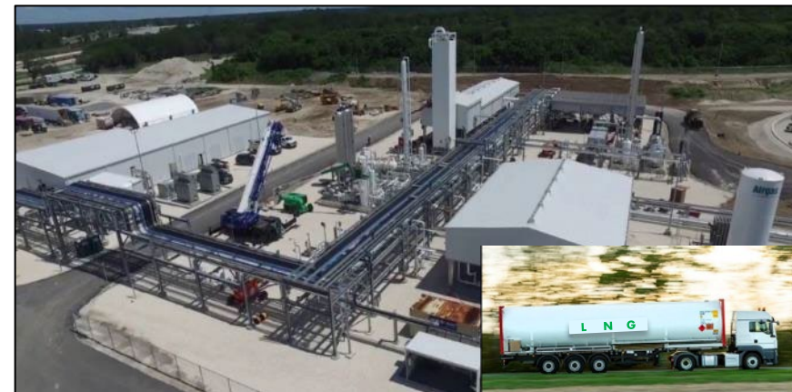
Modular LNG Plant –75,000 Tonnes Per Annum
